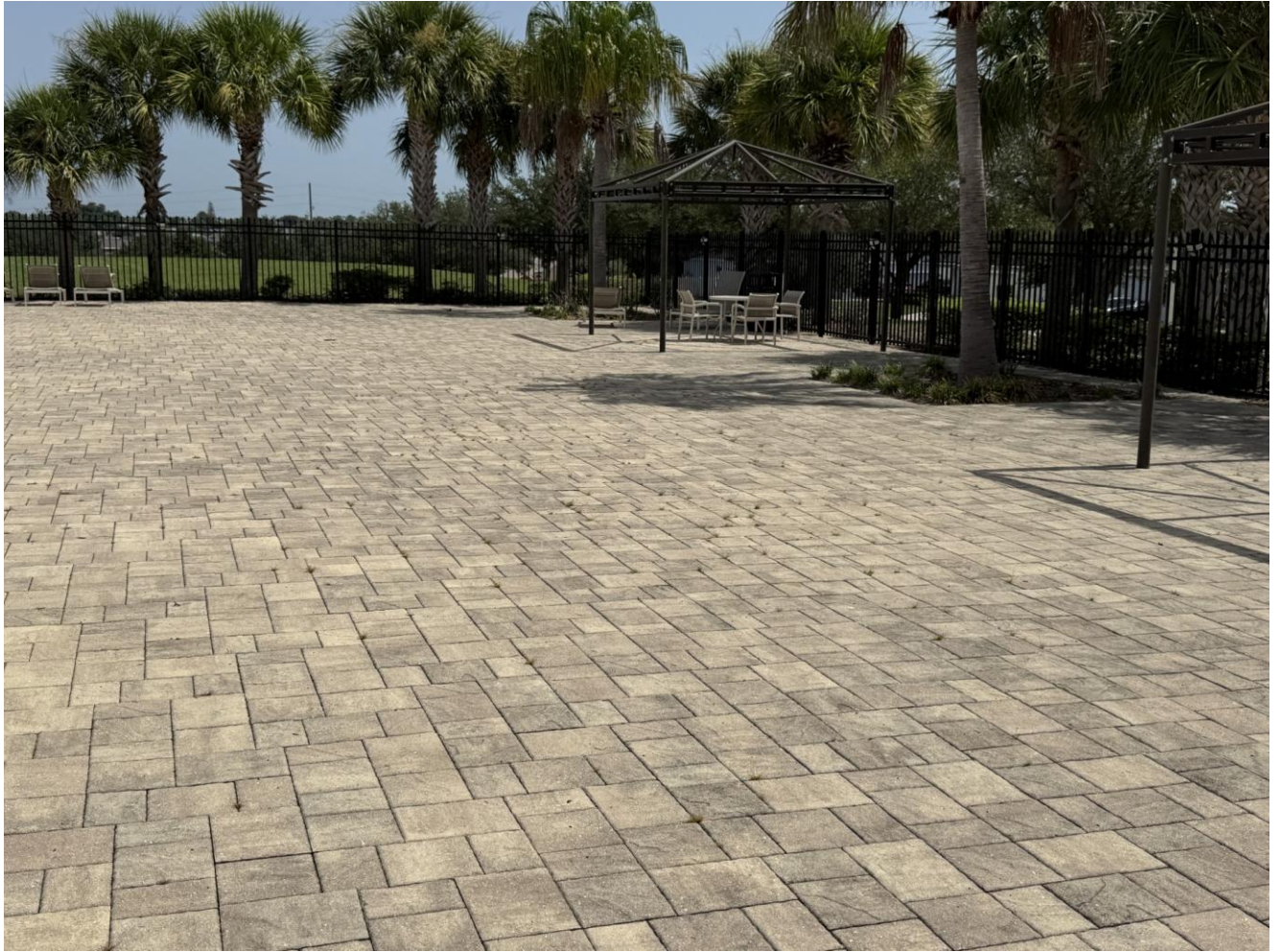
Small weeds present between pavers
